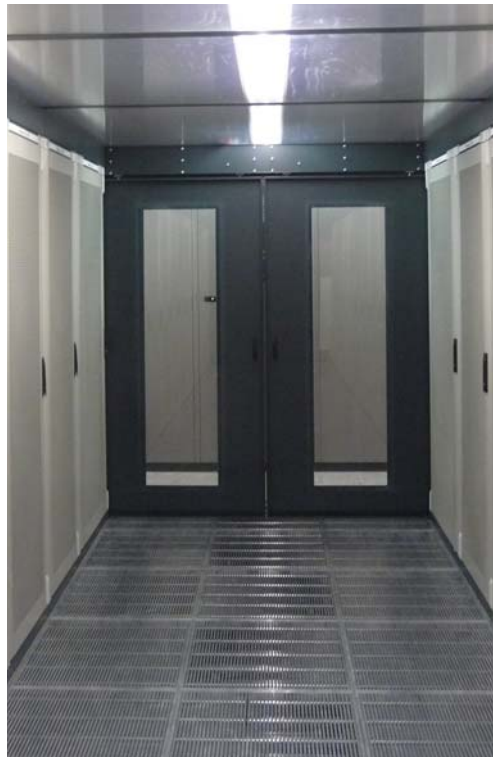
Example of a Cold Aisle Corridor
